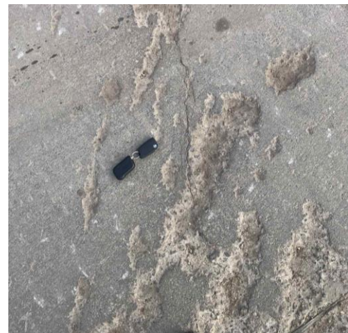
Figure 3. Damage to concrete pavement caused by direct shell hits
